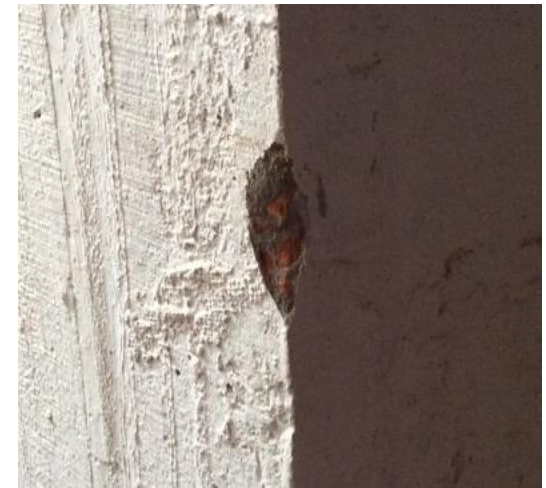
Tested Column – Brick Chips
