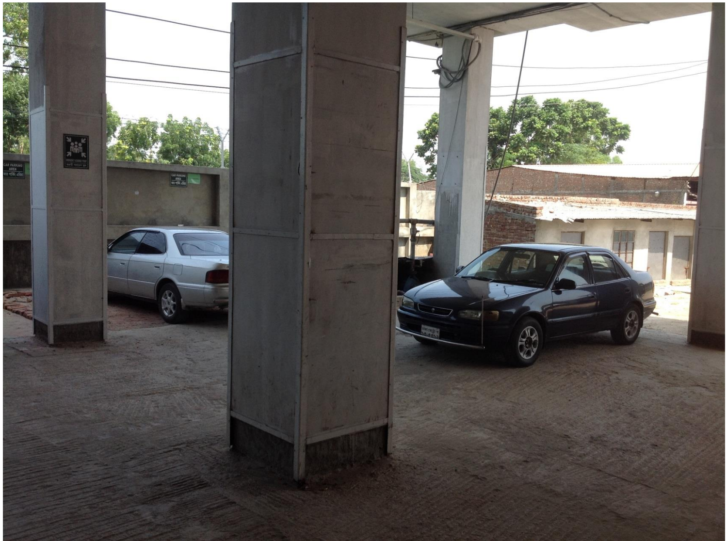
Columns at Loading Bay are susceptible to impact loading from vehicles.
