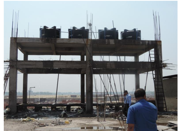
Water tanks on warehouse
