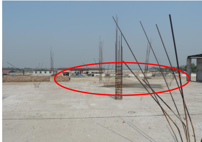
First floor parapet missing
