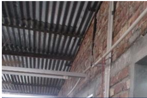
Roof shed without truss
