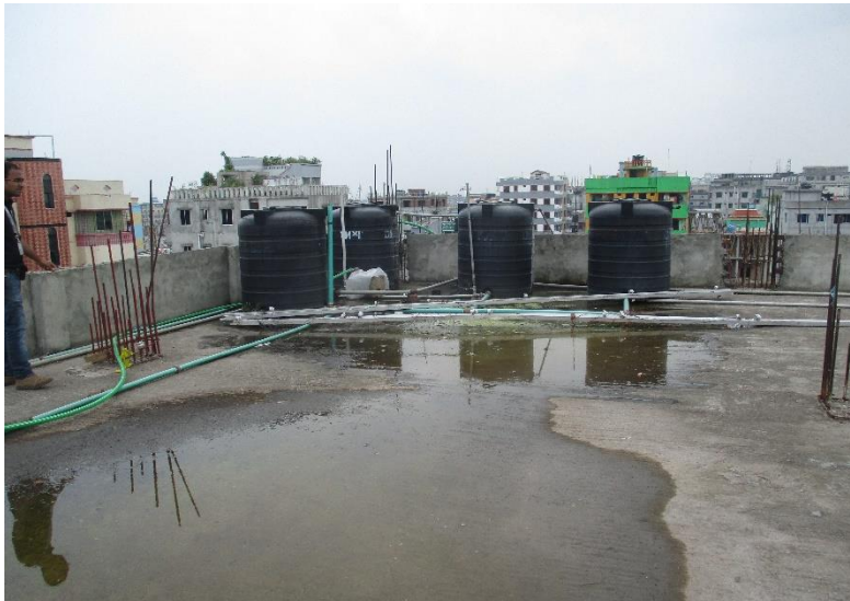
Water ponding at roof
