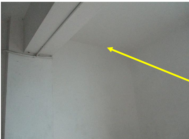
Cantilever at stair without beam
