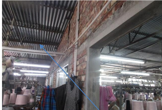
Roof shed without truss
