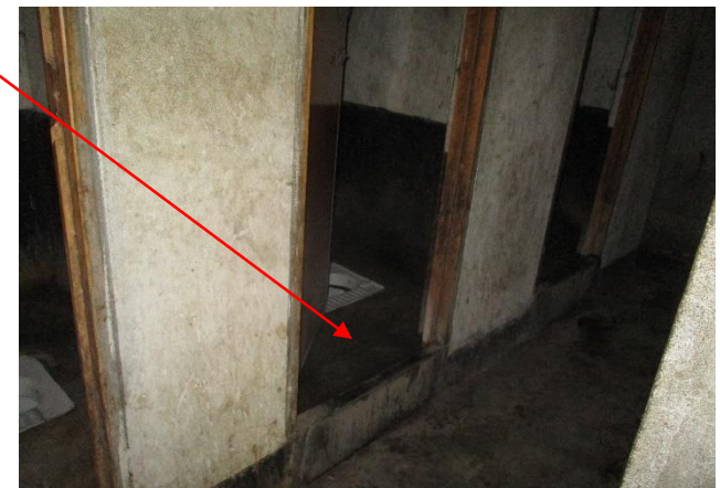
Toilet zone with build up
