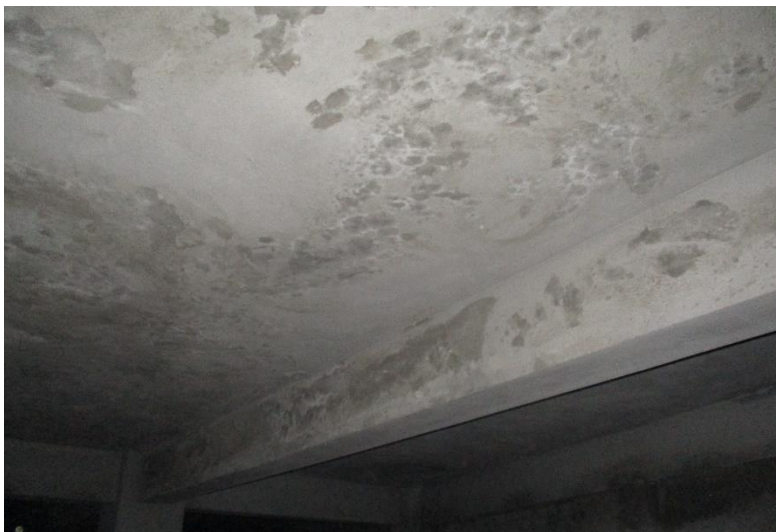
Water ingress at 4 th floor slab soffit
