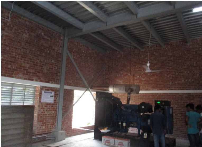
Generator & Sub-station building
