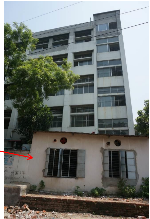
Single storey brick building on south side of main building. No record drawings. Building engineer to check.
