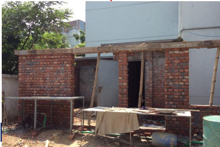
Brick building under construction on north-west side of main building. No record drawings. Building engineer to check.
