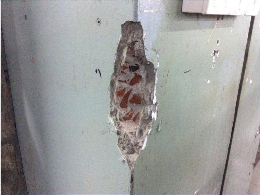
Brick aggregate exposed in columns on both sides of movement joint
