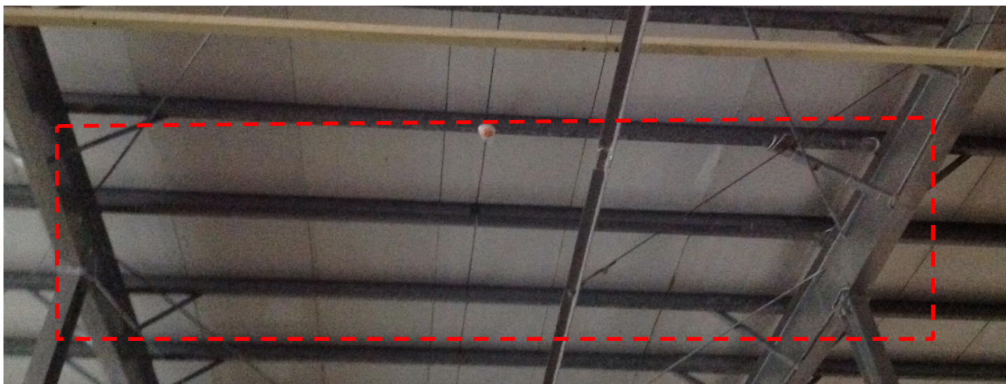
Compression Strut missing from roof bracing
