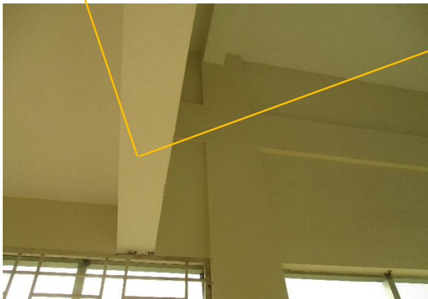
Beam shifted from drawings in yellow marked area.
