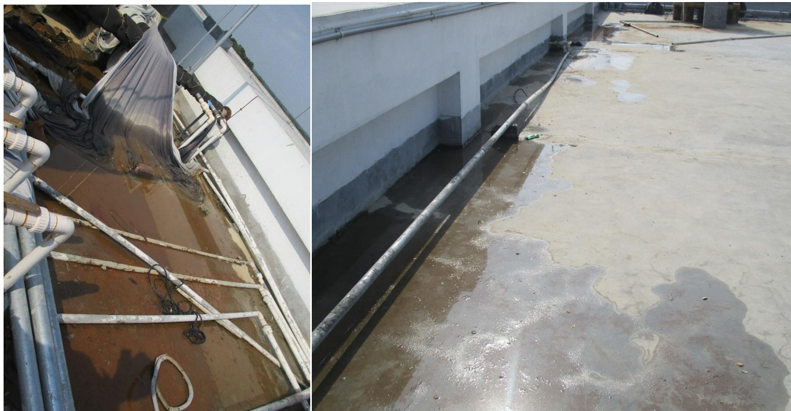
Poor water drainage system observed at roof of garments building.
