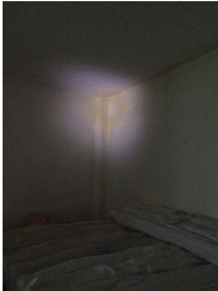
Leaking Toilet may allow water ingress to structural elements.
