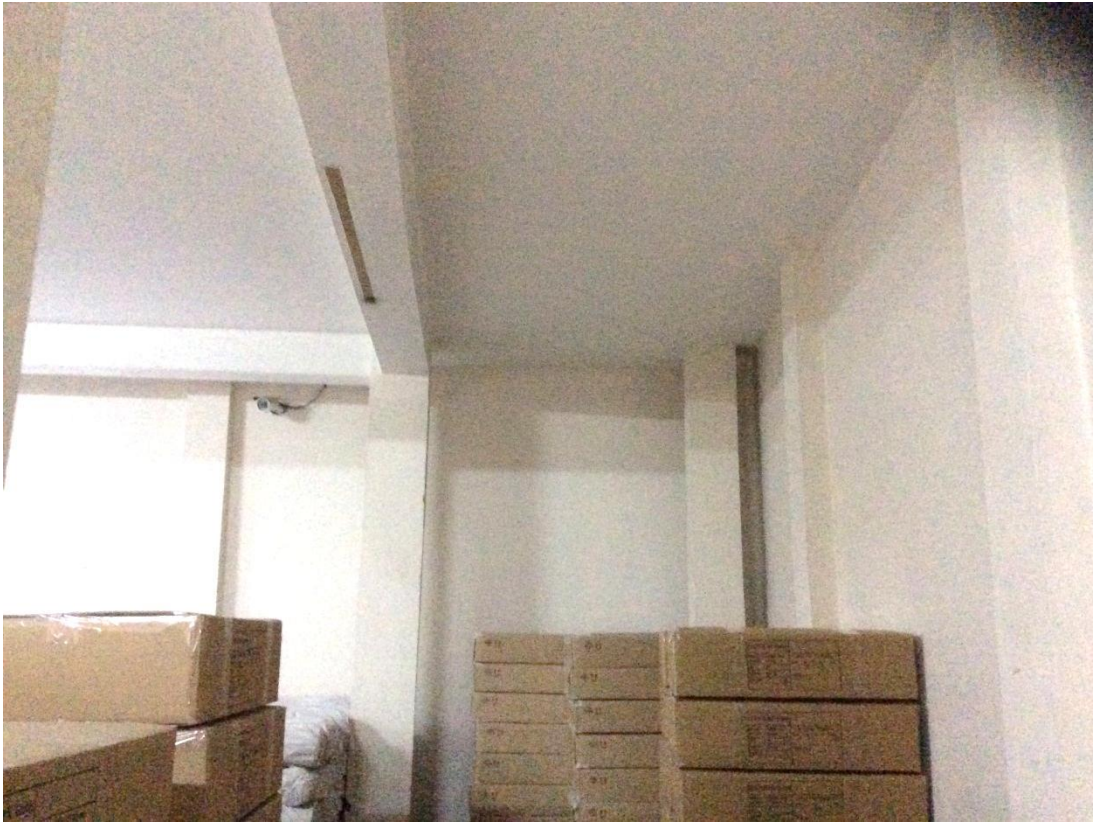
Cracks in soffits of slabs were recently decorated.
