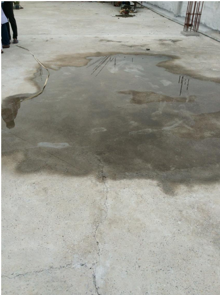
Cracking in roof finish may allow water ingress to structural elements.
