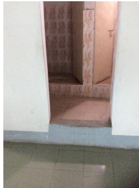
Large build-up in toilet area's on Cantilever slab.
