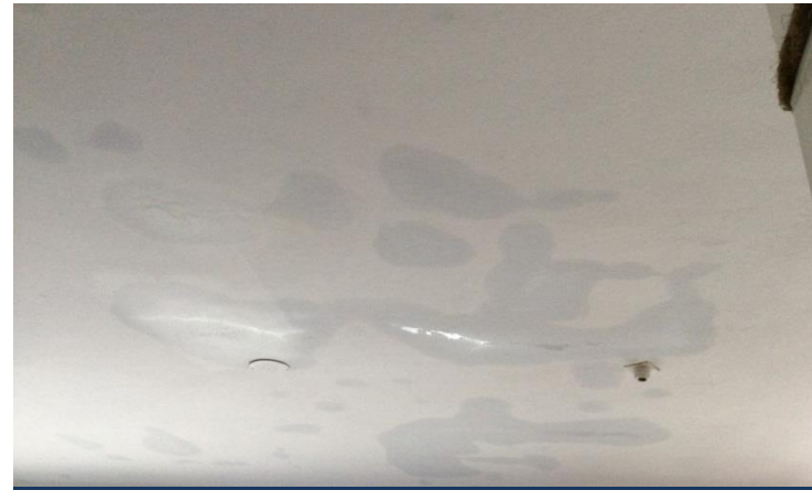
Cracking and water ingress in the soffit of the 6 th floor slab
