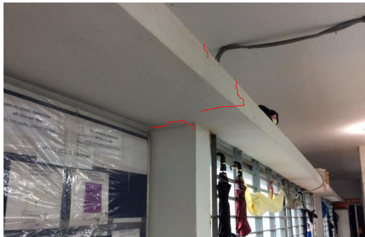
Cracks in façade on 4 th floor
