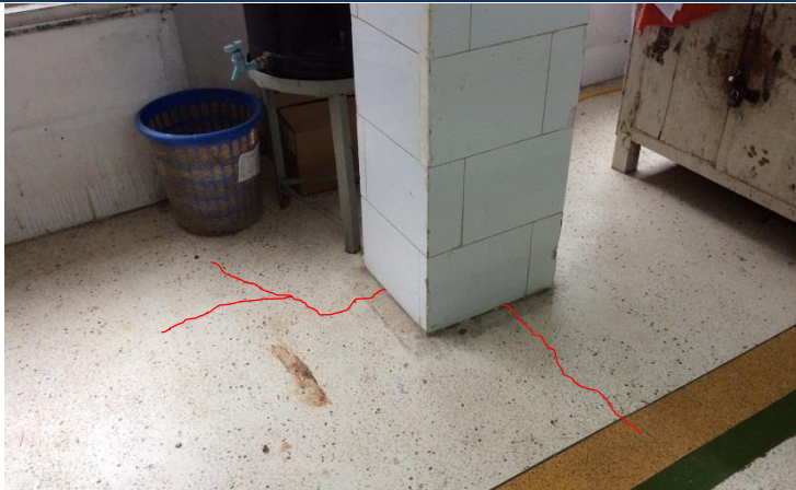
Cracking observed around column heads and along column strips
