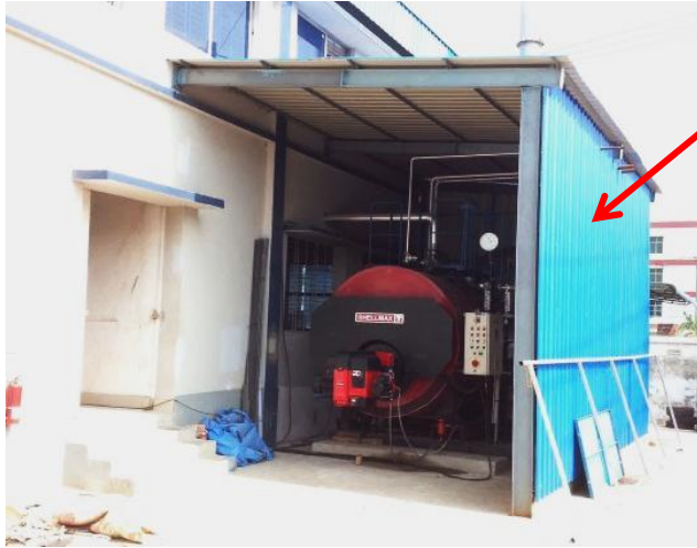
Generator room outside the building
