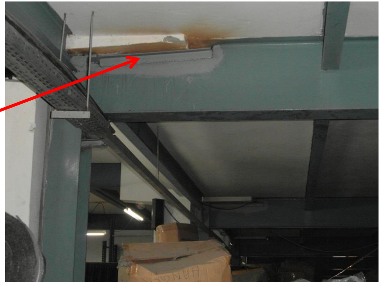
Top flange cut away and additional angle poorly welded with poor detailing – reduced flexural and shear capacity of beam
