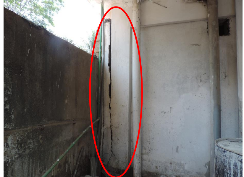
Separation of wall from building
