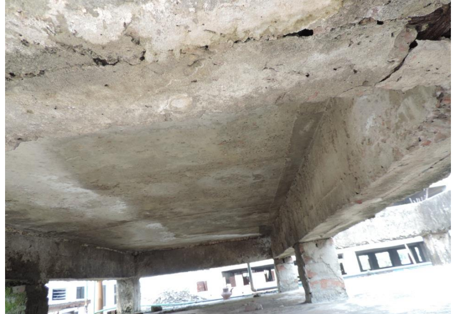
Soffit of water tank with concrete spalling
