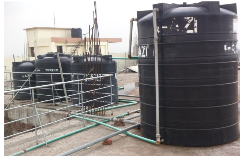
Water tanks on Level 7 (current roof)
