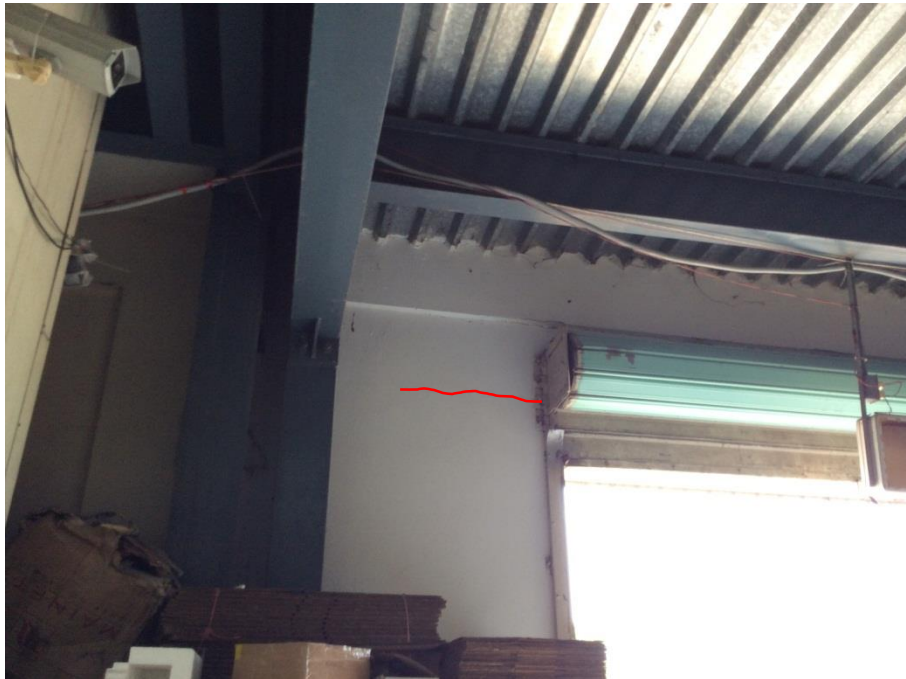
Cracking on ground floor
