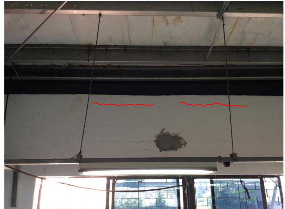
Cracking and signs of repairs on 1 st floor
