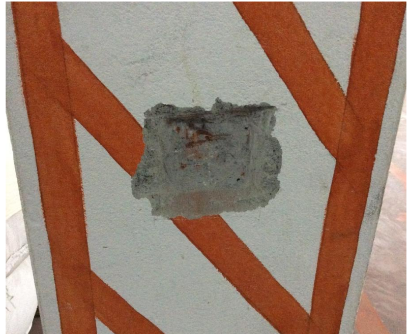
Brick aggregate in column
