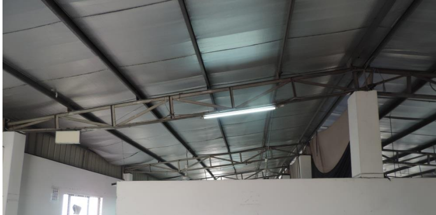
Lack of horizontal bracing in roof
