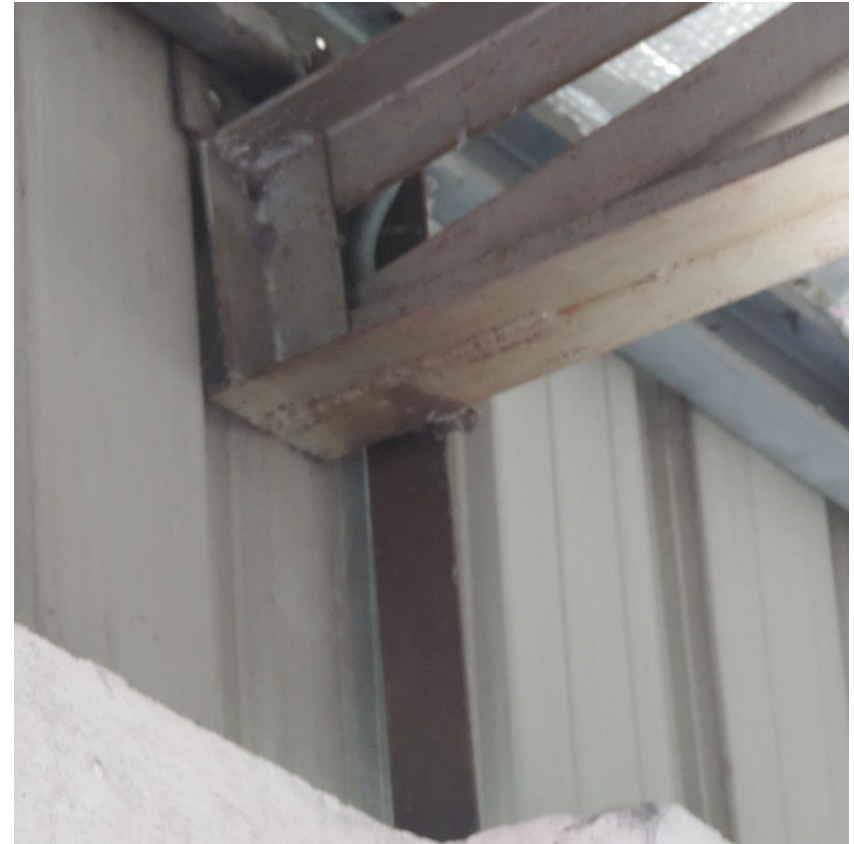
Non-engineered connection to column
