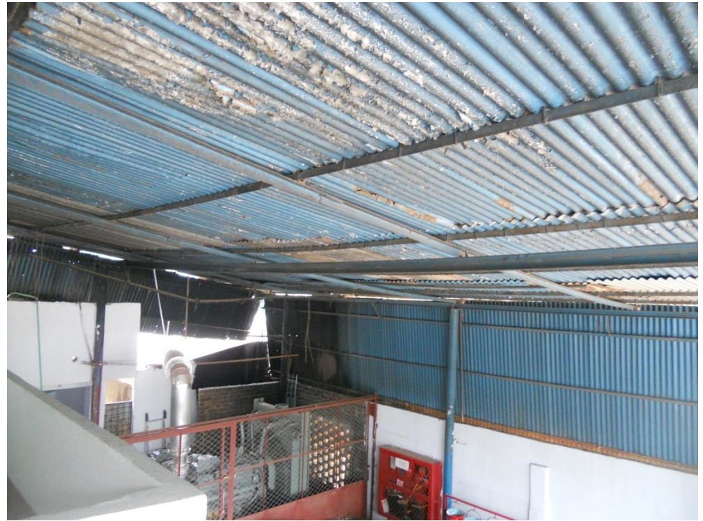
Roof to canopy at main entrance – deflection of roof supports.
