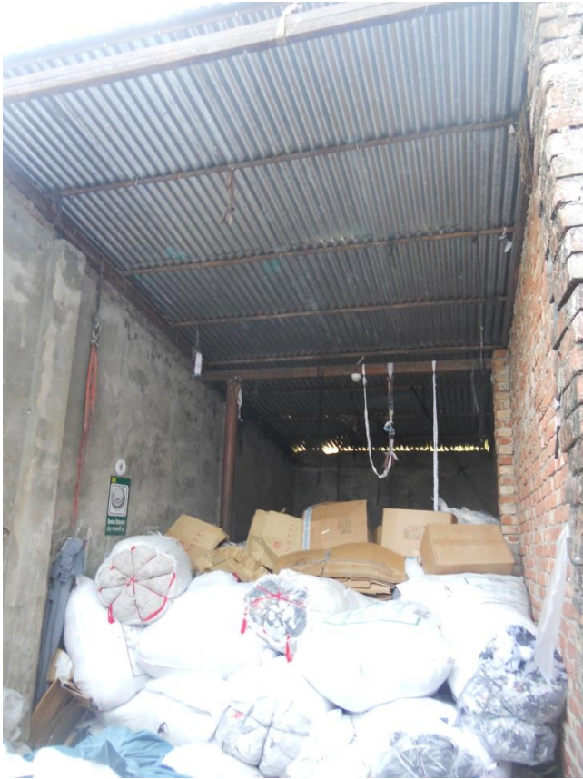
Waste Store Roof - sagging in roof beams.
