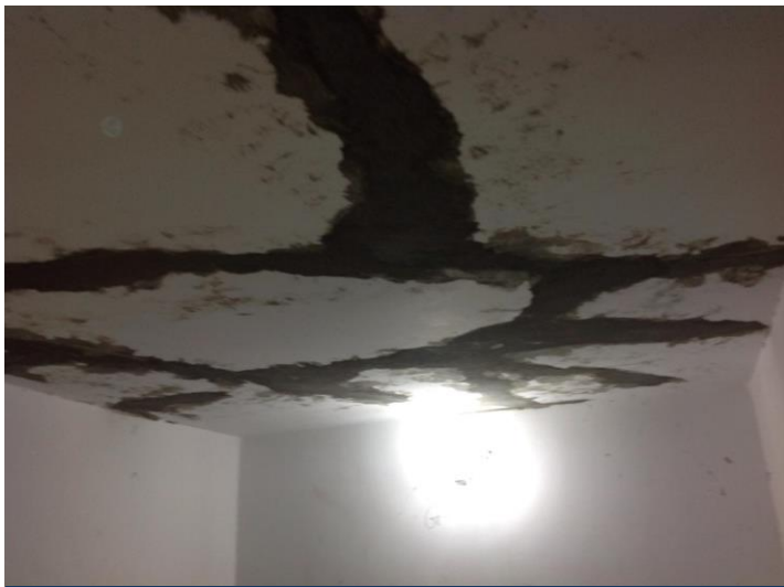
Evidence of distress on soffit of secondary ceiling slab (Building 1). Loading above not confirmed.
