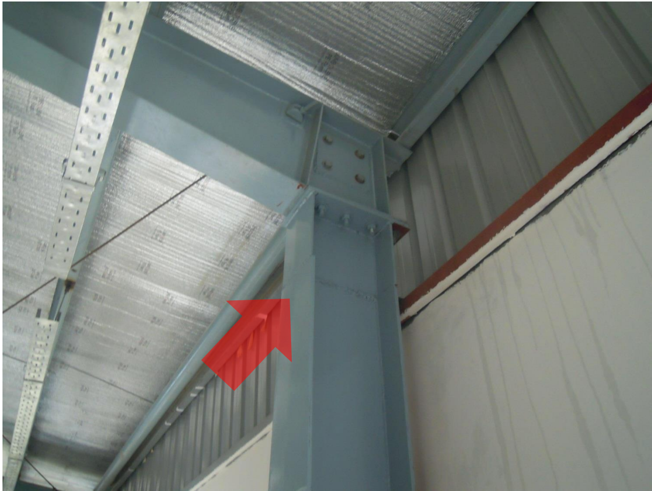
Change in column size was observed towards top of column in the new warehouse building
