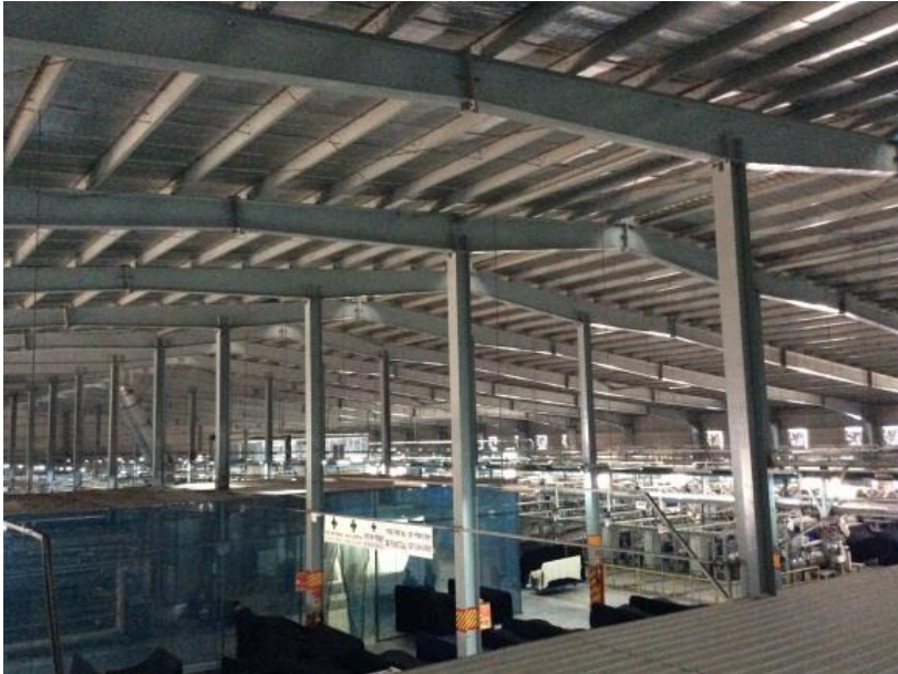
Typical Roof structure type observed in garment building, knitting building and dyeing building
