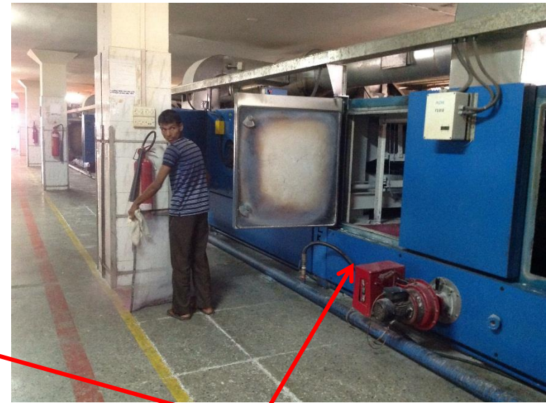
Stantar machines on ground floor – floor vibration noted
