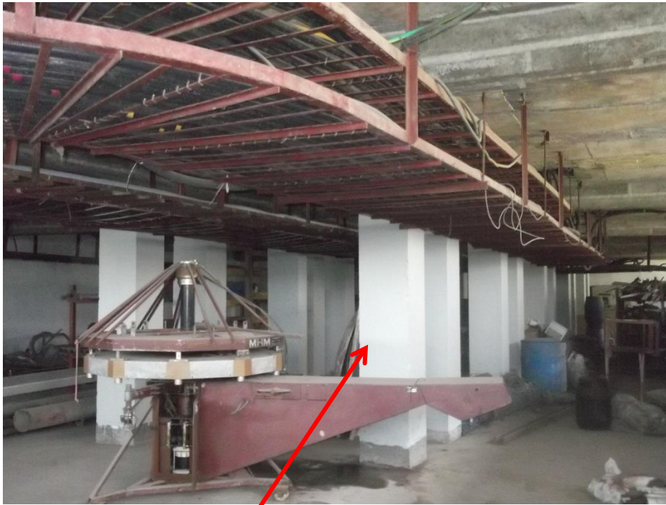
View of specific equipment support columns within the basement of the Utility Building
