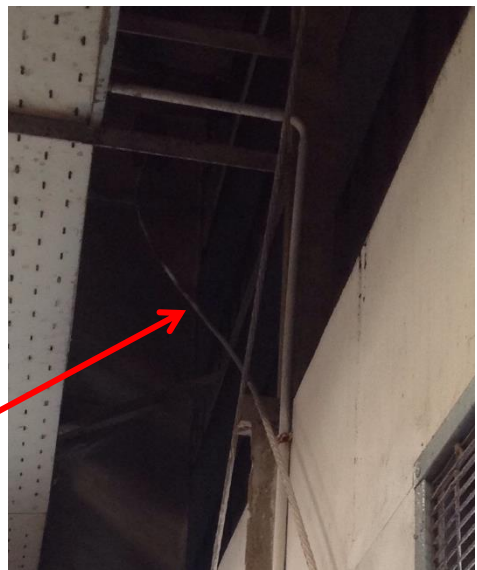
Damaged bracing to be reinstated
