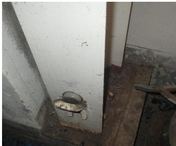
Corroded steel column at support.
