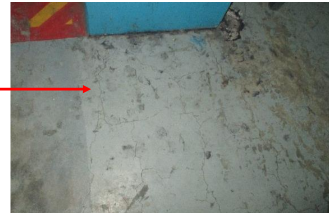
Cracking to soffit of 1 st floor slab
