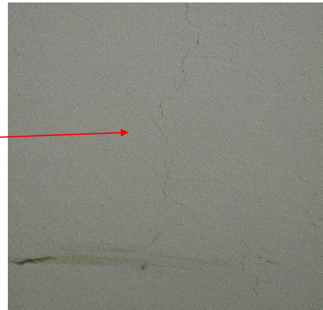
Cracking to soffit of 1 st floor slab
